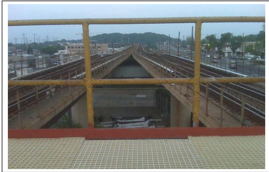
Picture 3 - D & G Platform facing Benning Road portal and Minnesota Avenue aerial structure.
